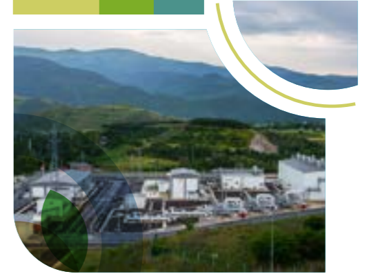
Metering Station (MS-1) Ardahan
