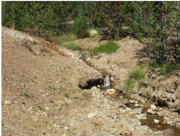
Figure 2.12 Undercutting of the riverbank at KP 616+207
